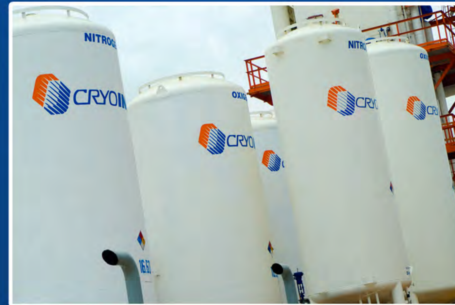
Liquid Backup Tanks
